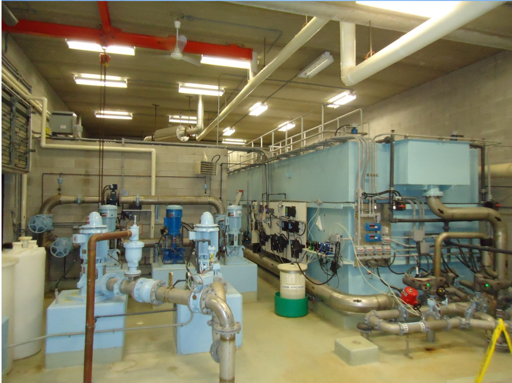
WARKWORTH WATER TREATMENT
